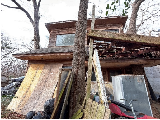
(Photo# 65 taken 2.25.26 by KK. Photo taken of the collapsing deck, trash, and debris around improvement #2.)
