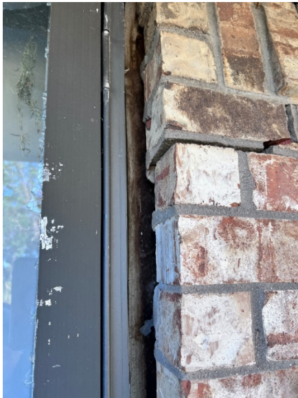
3. Large crack on East side – wide enough to fit a hand in vertically
