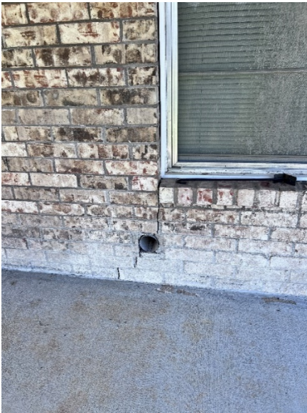
3. brick falling away from the structure, exposed wiring
