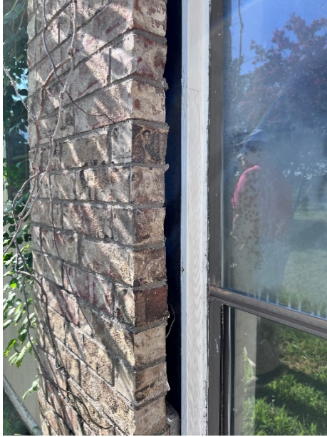
2. Brick falling away from structure around window
