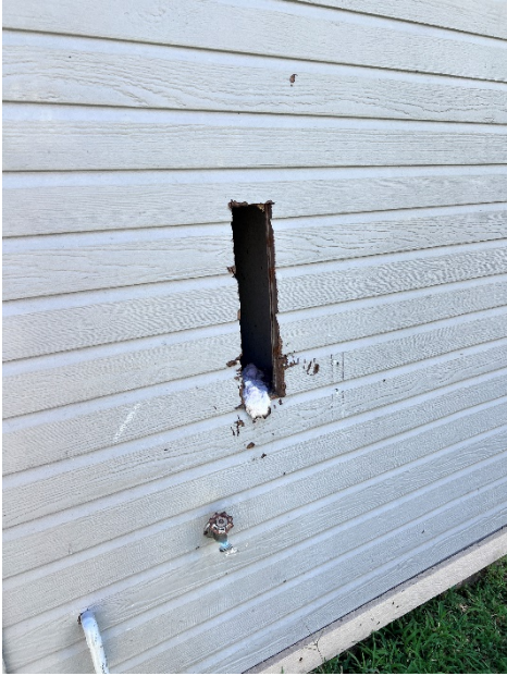
2: Unknown exposed open conduit into the building
